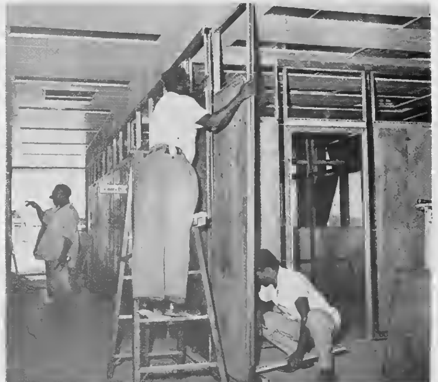
PUTTING up flexible birch partitions to form office walls was fairly simple. PONEMENTO di particionnan flexible di berk pa forma muraya tabata facil.
